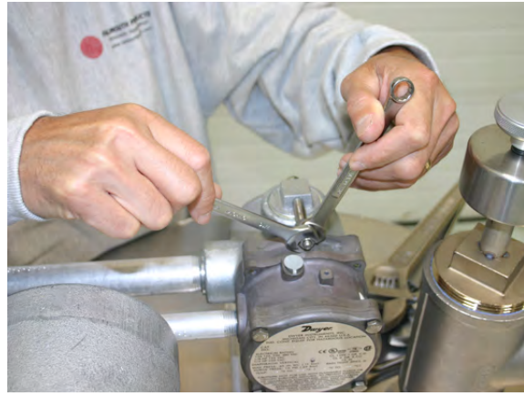
Unbolt the pressure switch with two 7/16” wrenches.
