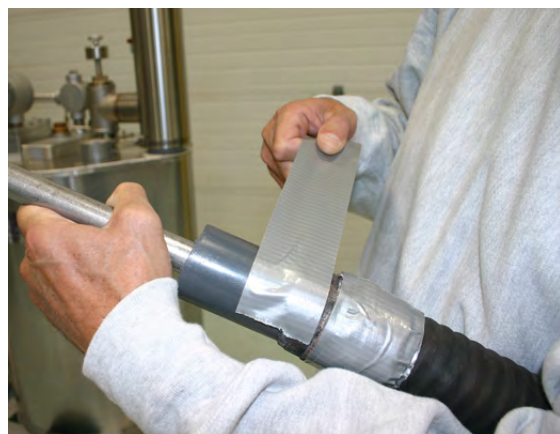
Prepare a shop vacuum with 48” piece of 3/4” tubing. Use 3/4” Electrical Metallic Tubing (EMT). Duct tape the tubing to the end of the vacuum hose.
